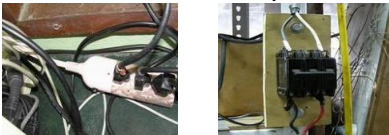
Unsafe electric facility
